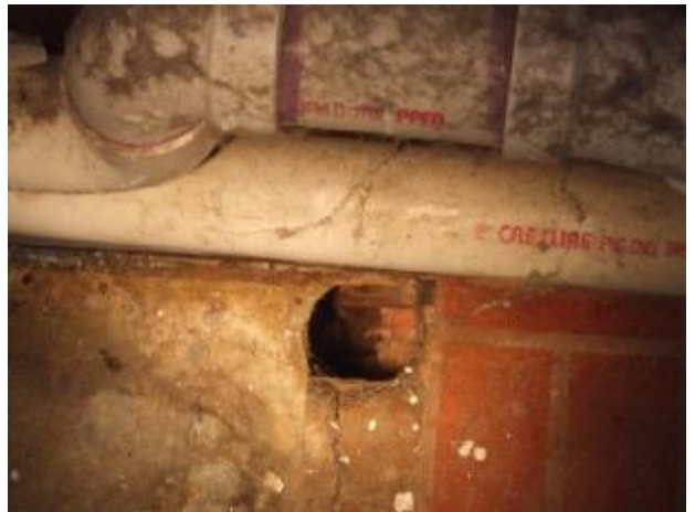
Hole in the floor. Possibly a former water discharge line.
