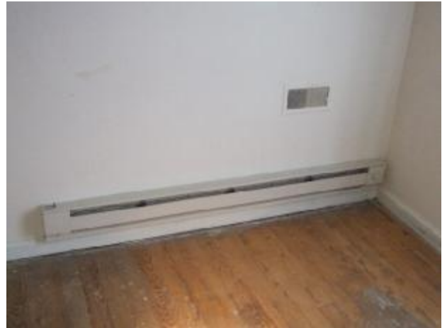
This baseboard heater is not working.
