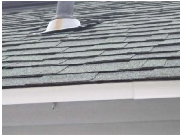
This vent is loose. Water can infiltrate.
