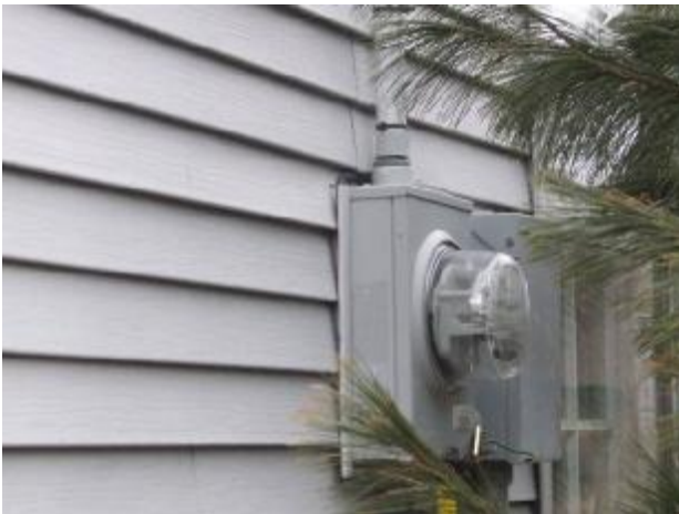
Electrical meter is here.
