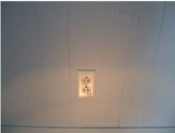
Broken receptacle covers should be replaced.
