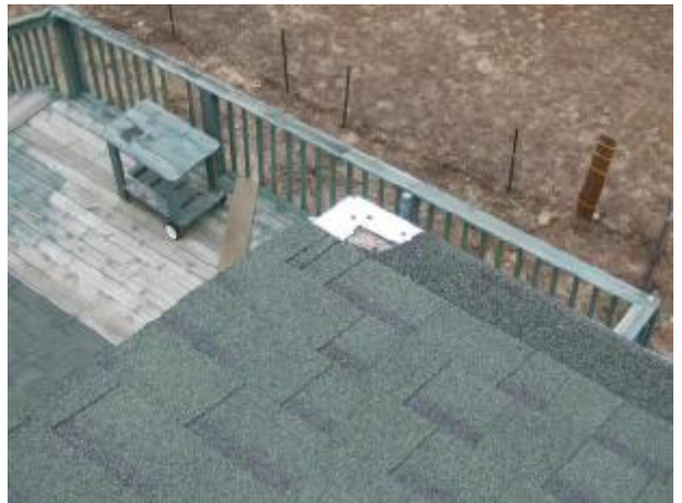
Shingle missing on the corner
