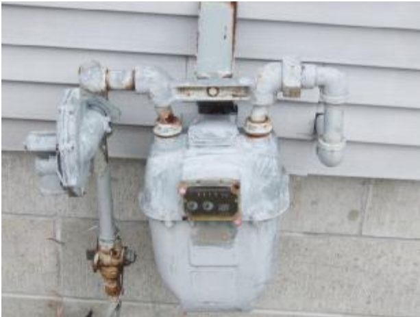
The gas meter is on the end of the house.
