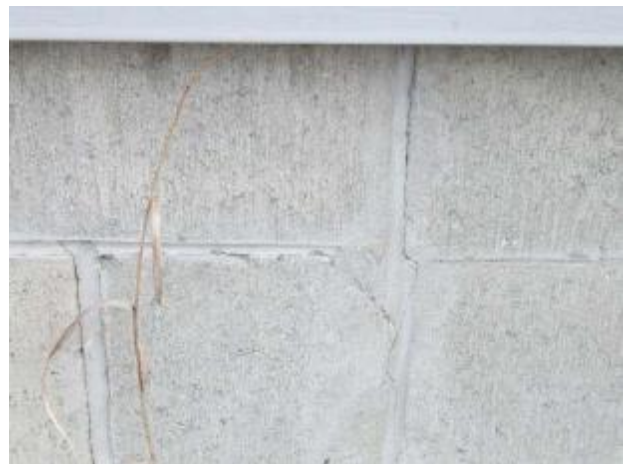
Loose grout is evident on the foundation.
