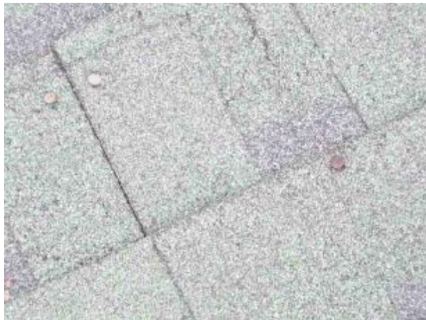
Several nails pounded into exposed shingles
