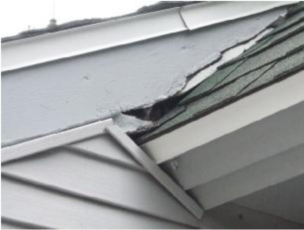
This hole really needs to be fixed. Water infiltration is imminent.
