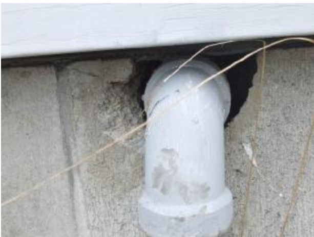
This vent pipe needs to be filled in.
