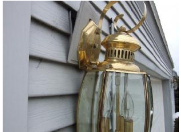
This fixture is loose and should be reattached.
