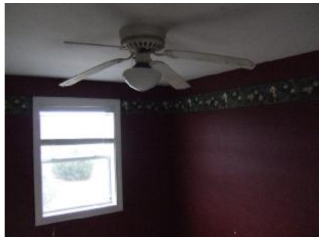
Neither the light nor the fan were operable in this room.
