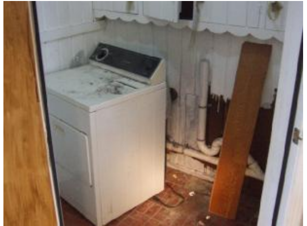
The dryer is set up for gas.
