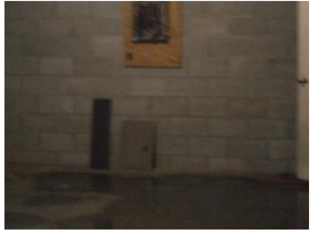
The electric service panel is located above a standing water issue.
