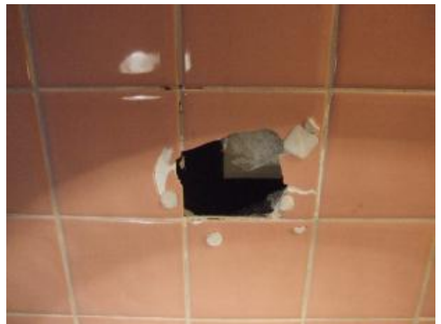
This tile needs to be replaced.
