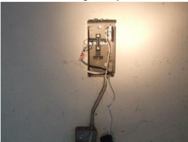
Exposed wiring needs to be cleaned up.
