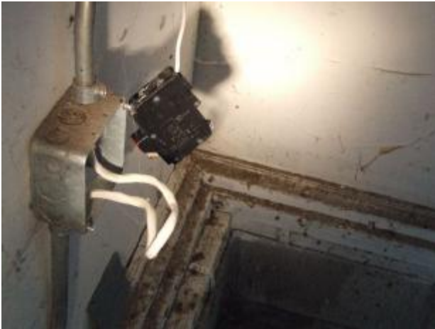
This wired up breaker is hazardous.
