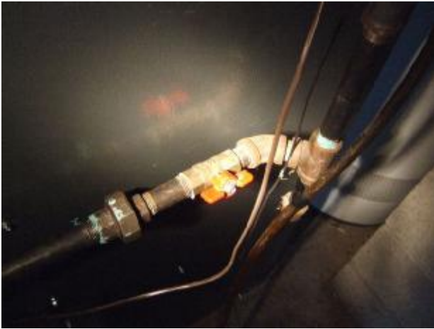
Gas shut off is located on the side of the furnace.
