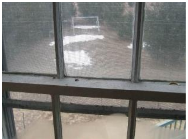
Upstairs room over the deck. Neither window has a locking mechanism.
