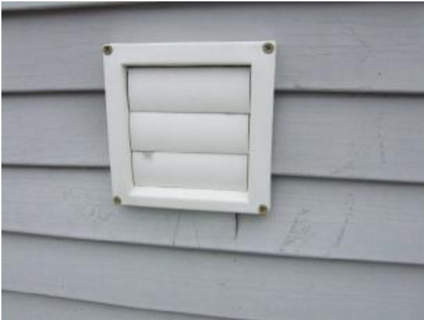
Cracked siding below this dryer vent.
