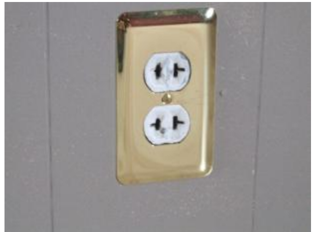
Several old outdated receptacles still exist.
