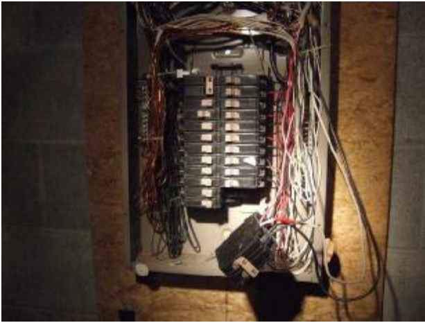
The panel appears correctly wired, however, this breaker hanging out is dangerous.
