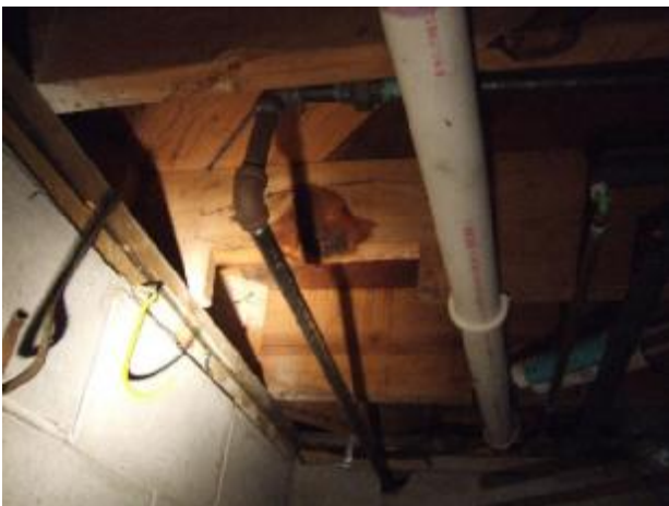
The integrity of this joist is questionable. A lot of wood was cut away for the gas line.
