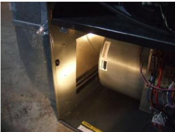
Furnace filter is missing.
