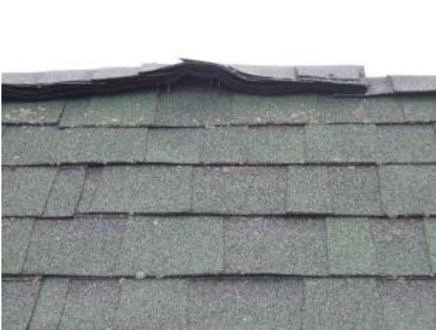
Ridge vent is loose
