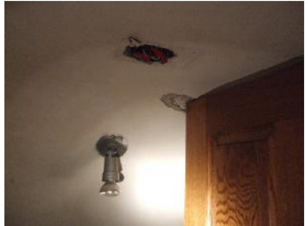
Exposed wires, the ceiling had to be dug out to accommodate the door as well.
