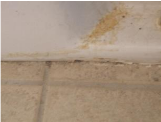
This toilet should be re caulked.
