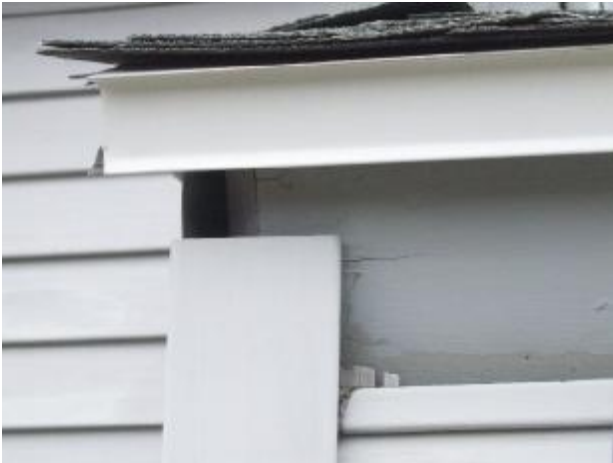
A large gap in the trim.
