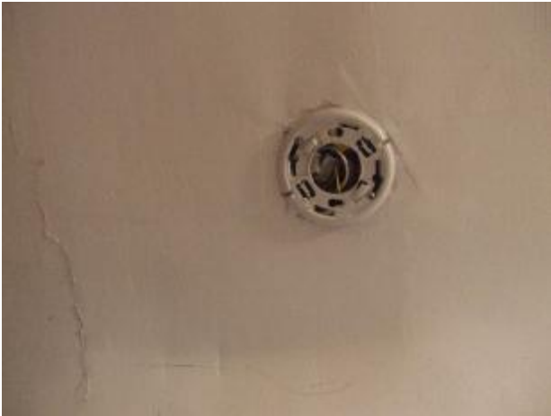
Fire alarm is missing.
