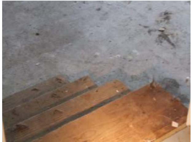
A railing would provide a safer entrance/exit to the house./
