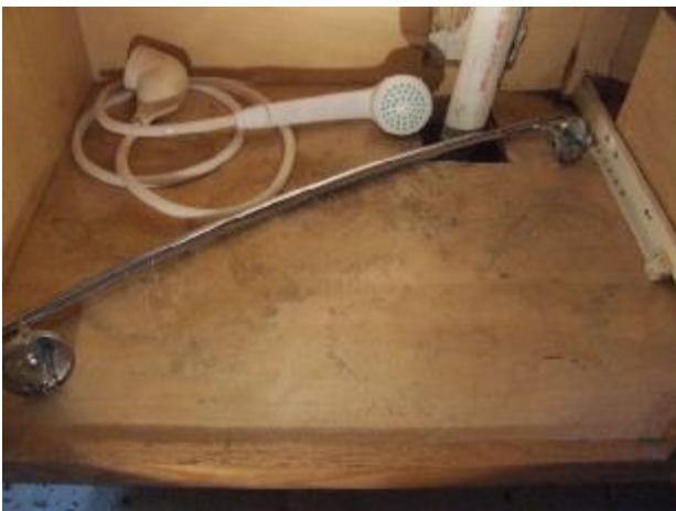
The rippled wood in the bottom of this cabinet is from standing water.
