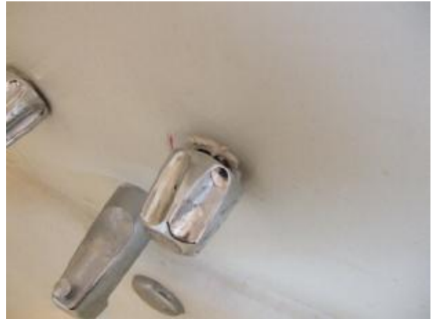
I am not sure why this was caulked.
