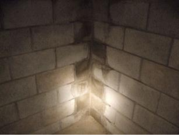
Damp foundation wall.
