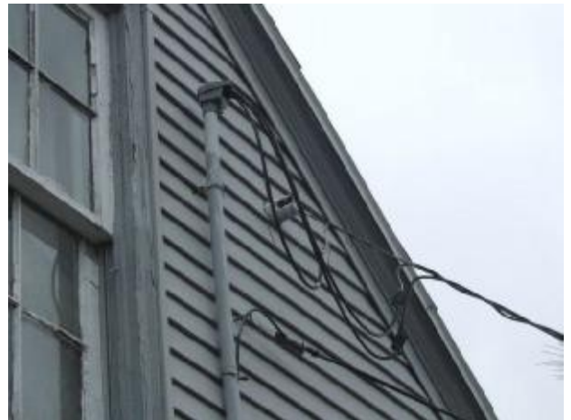
The electrical service mast looks good and the wires droop to help keep out water.
