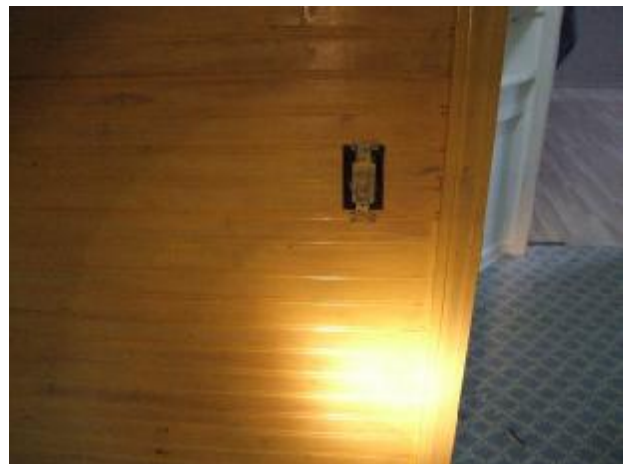
All outlets and receptacles need covers.
