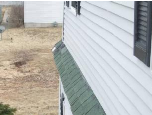
Missing shingles at the end of this eve.
