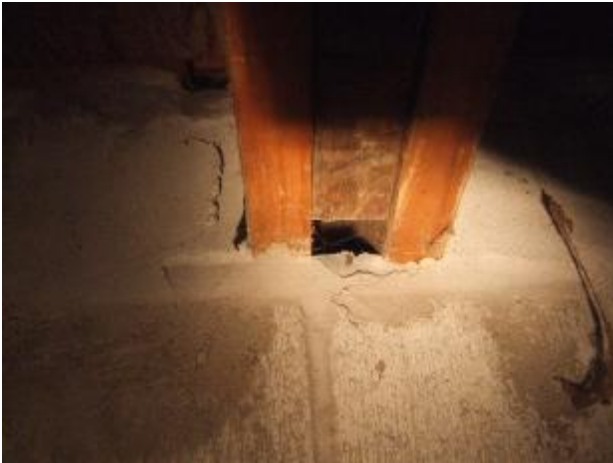
This hole should be patched.
