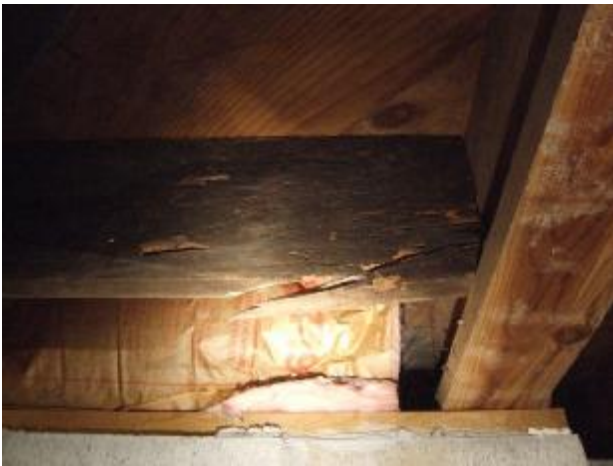
Broken joist should be replaced.
