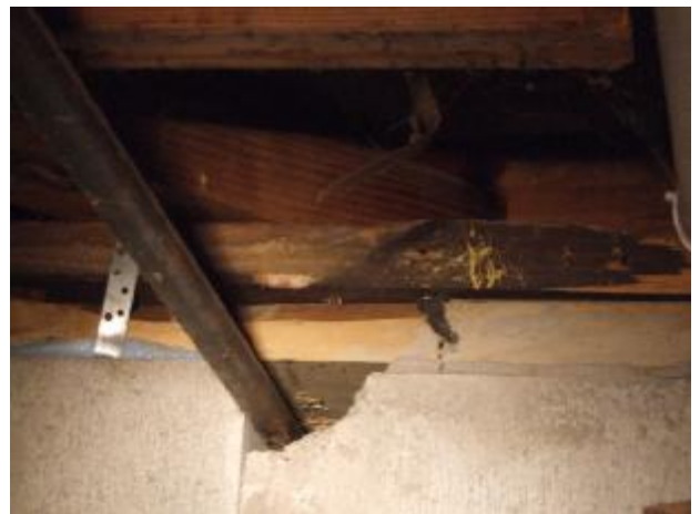
This hole should be filled.
