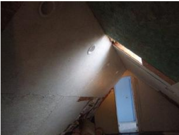
The lights in this room are not working, and the exposed insulation should be covered.
