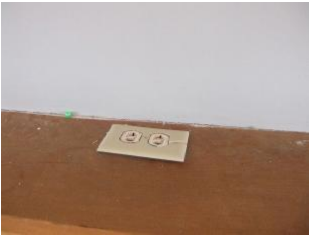
Loose and old wiring on the mantle.
