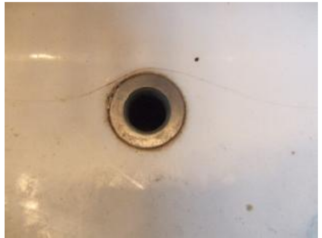
The line you see is a crack in the sink.
