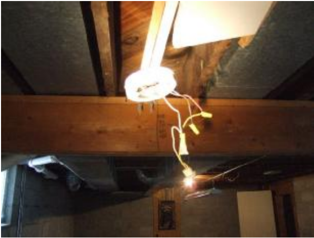
Exposed hanging wires are not safe.
