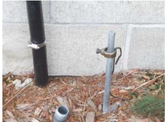
Electrical grounding rod is located here.
