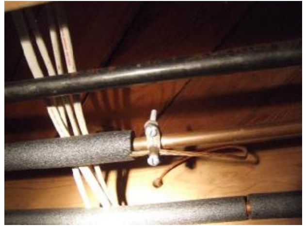
Electrical ground to the water line.
