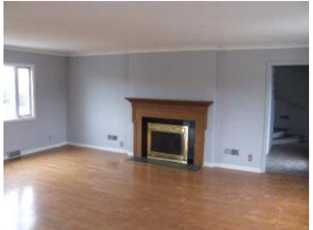
The fireplace is loose.
