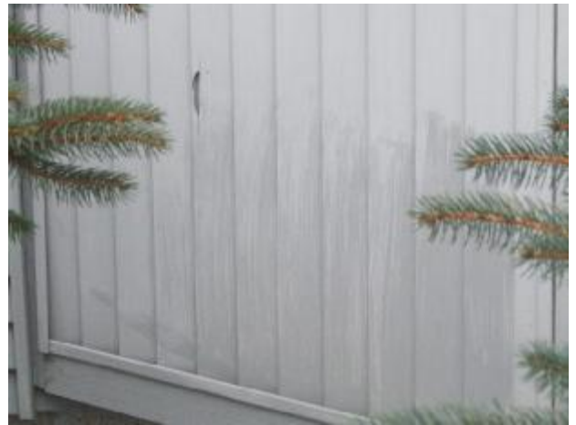
The siding has been painted. The holes should be patched.
