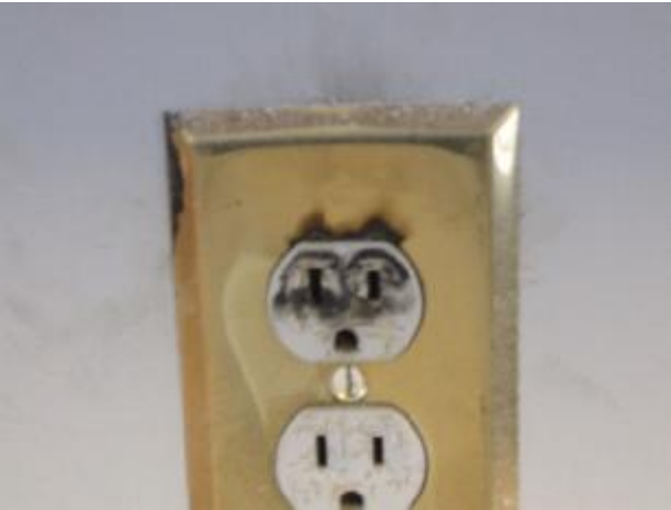
This receptacle has obviously overheated. It should be replaced.
