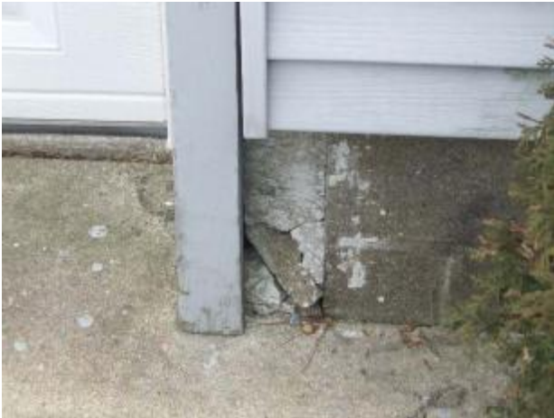
Broken, crumbled block at the garage door.
