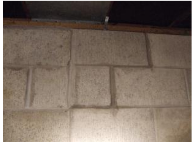
The foundation blocks with the dark lines appear to have been re-grouted.
