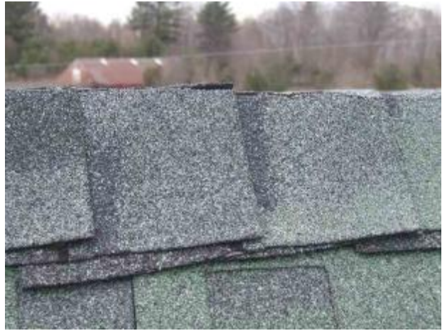
Cracked, broken shingles on roof cap.
