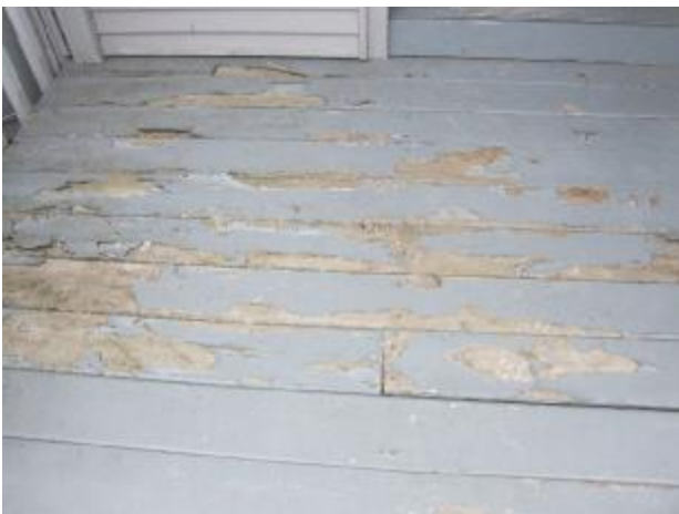
The front porch paint is flaking and should be scraped and repainted.
