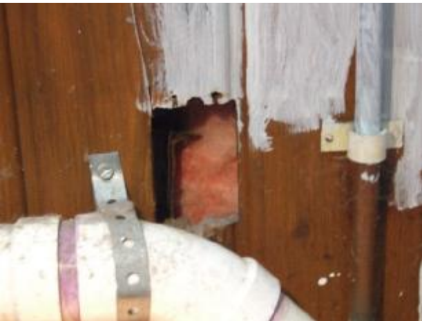
An electrical box formerly occupied this hole.
