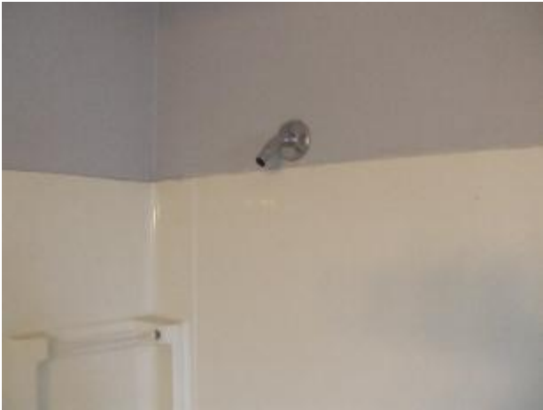
Shower head needs to be installed.
