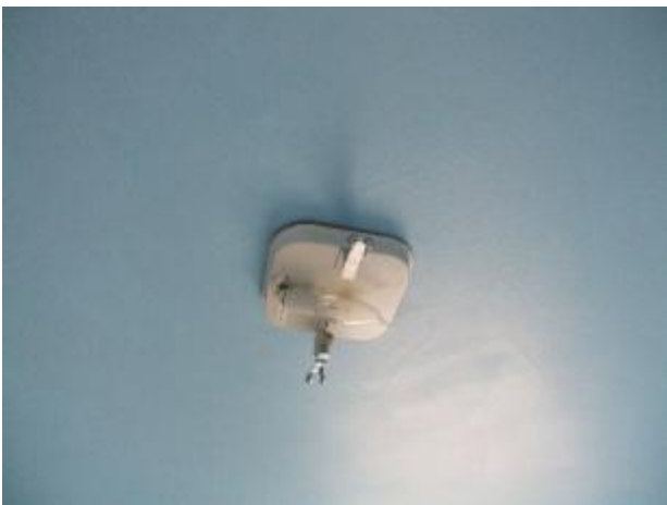
This fixture should have a cover on it.
