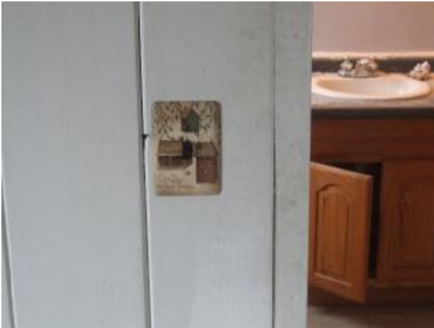
This switch is not properly working and needs to be replaced.
